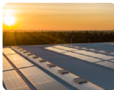
Solar Powered Warehouse Panels
